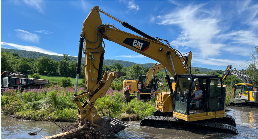
An excavator adds wood to a Blakeslee Preserve stream during the restoration project in August 2022. © Su Fanok/TNC
