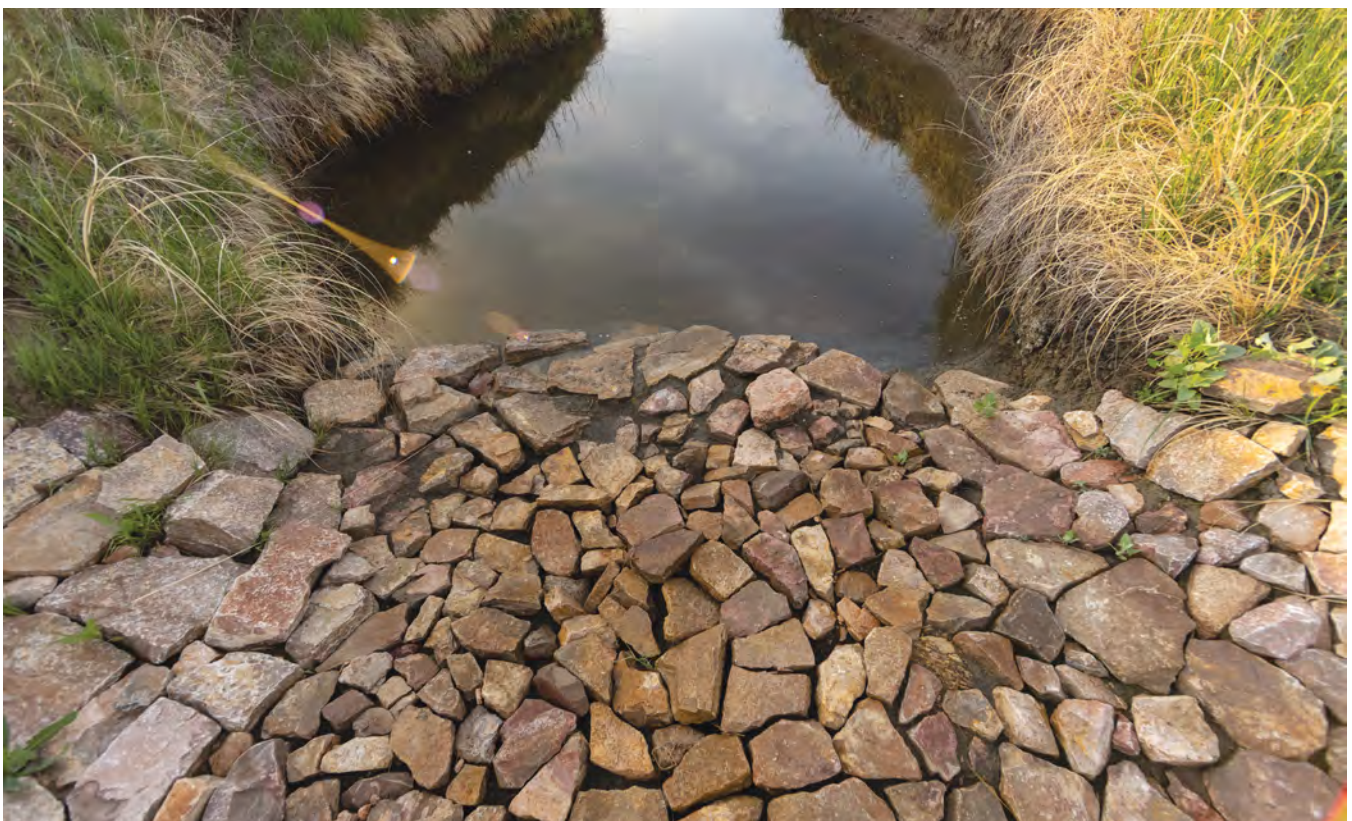
Figure 94: Zeedyk structures are used to prevent advancing headcuts and incision. These photos show a larger headcut that was “laid back” and covered with a Zeedyk rock structure. The rocks work to trap sediment from upstream. Root growth and vegetation will establish within crevices, allowing the site to heal. Photos © Joe Dickie, Generation Photography, Inc.
