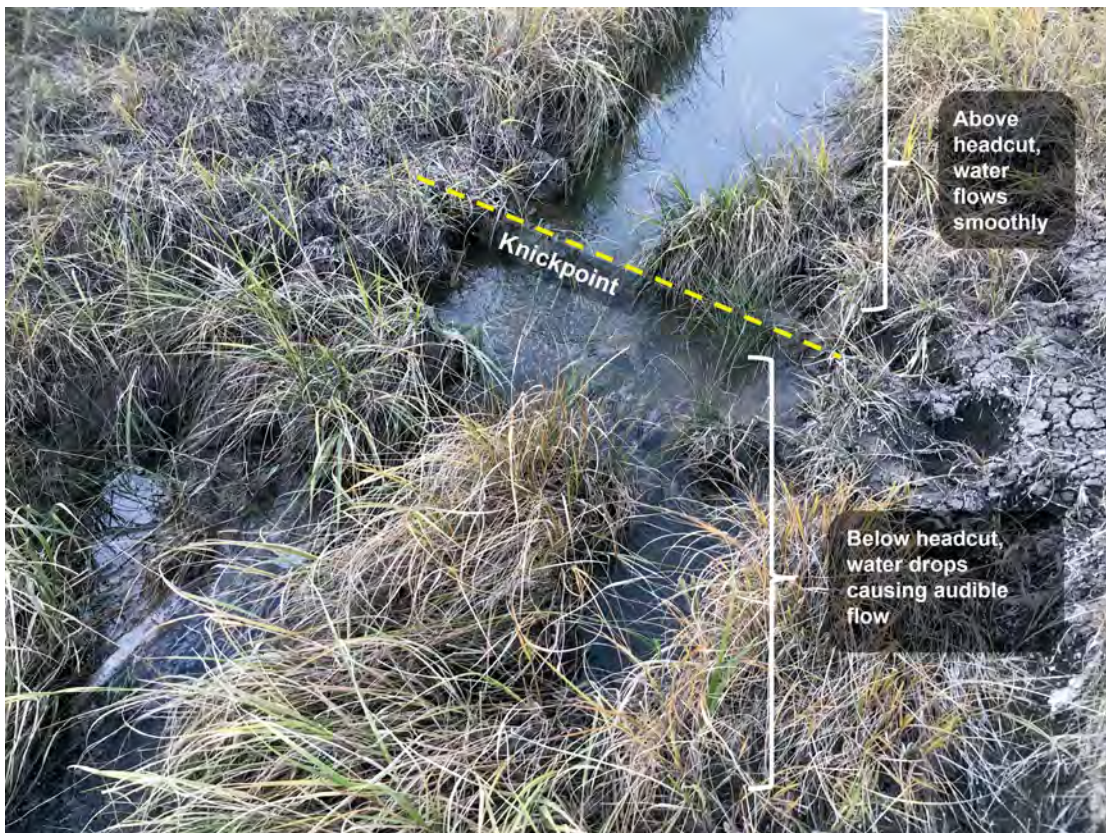
Figure 81: When headcuts occur below water, they may not be easily visible—but they often can be heard. Here, the knickpoint where a headcut is forming underwater causes the water level to drop. The rush of water flowing down is audible. Photo © Corissa Busse, TNC
