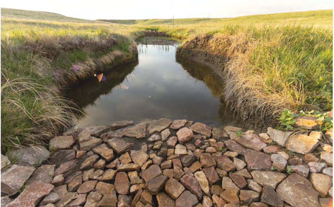
Figure 2. A Zeedyk rock structure installed to help prevent headcuts from eroding upstream reaches. Photos © Joe Dickie, Generation Photography, Inc.
