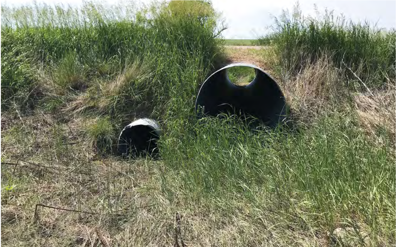
Figure 91: Culverts and road crossings can significantly constrict the flow of water in a stream during flood events. This constriction point can then intensify the force of waters, creating headcut and incision challenges, which not only create challenges for the stream but also compromise the road over time. Photo © Christian Lenhart, TNC
