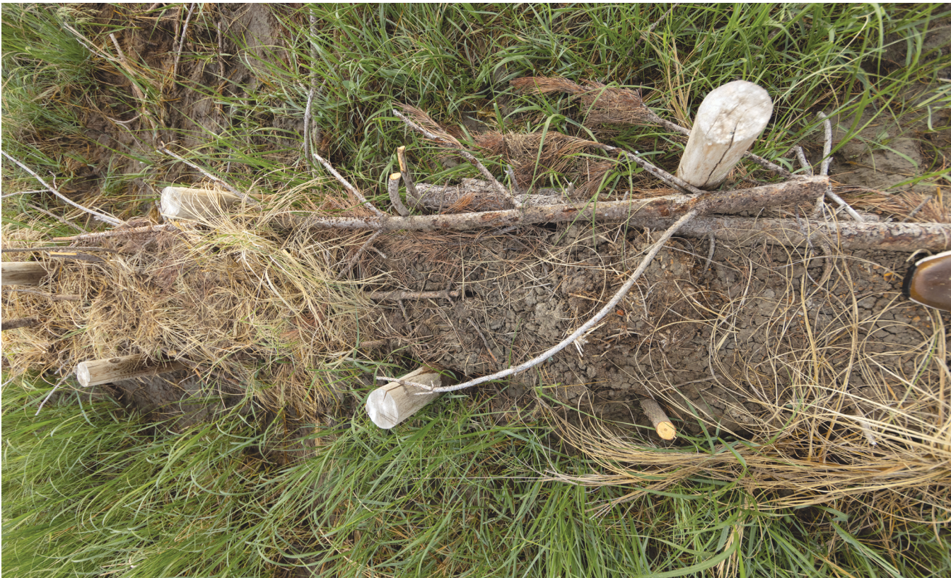
Figure 97: These images show a side and top profile view of a beaver dam analogue. BDAs use local materials, including sod, grasses, or woody vegetation woven between and secured in place by untreated wood posts. Photos © Joe Dickie, Generation Photography, Inc.
