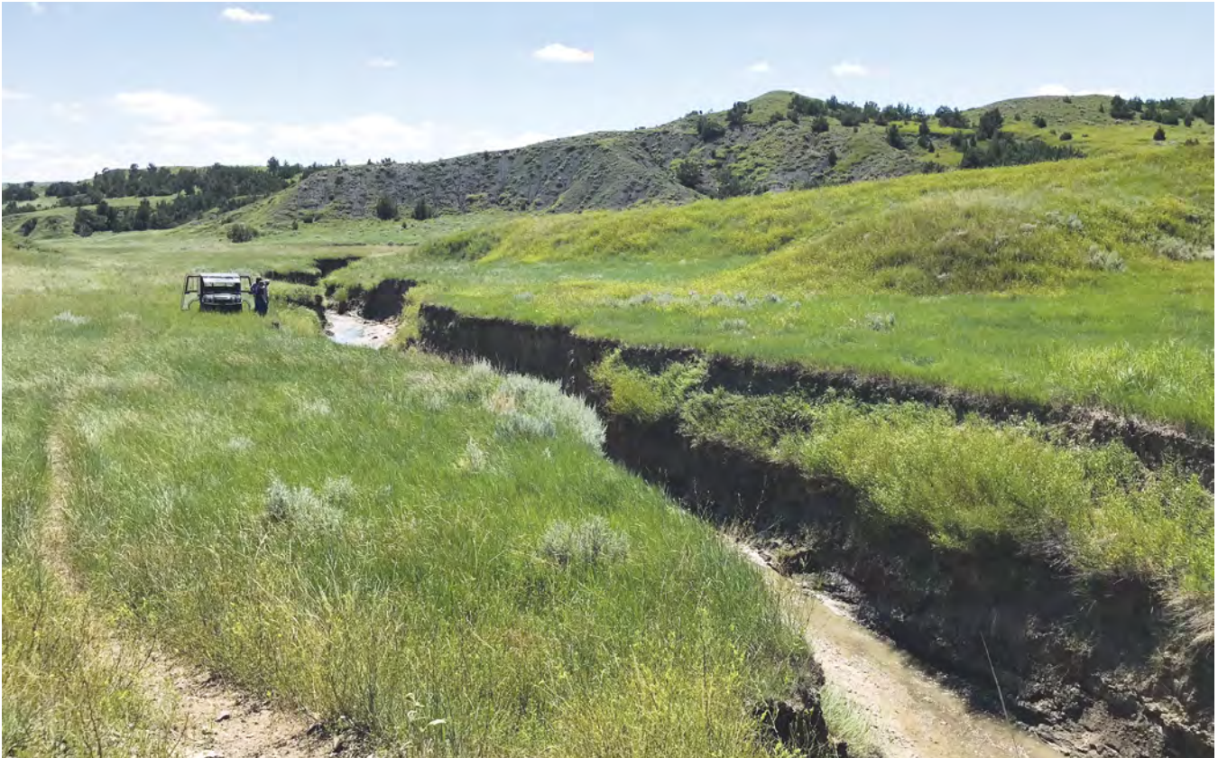
Figure 82: This stream has incised nearly 10–15 feet. It is no longer easily crossed or accessible to livestock and wildlife. The surrounding meadow area will lose vegetation productivity due to the drop in the water table. Photo © Kristen Blann, TNC
