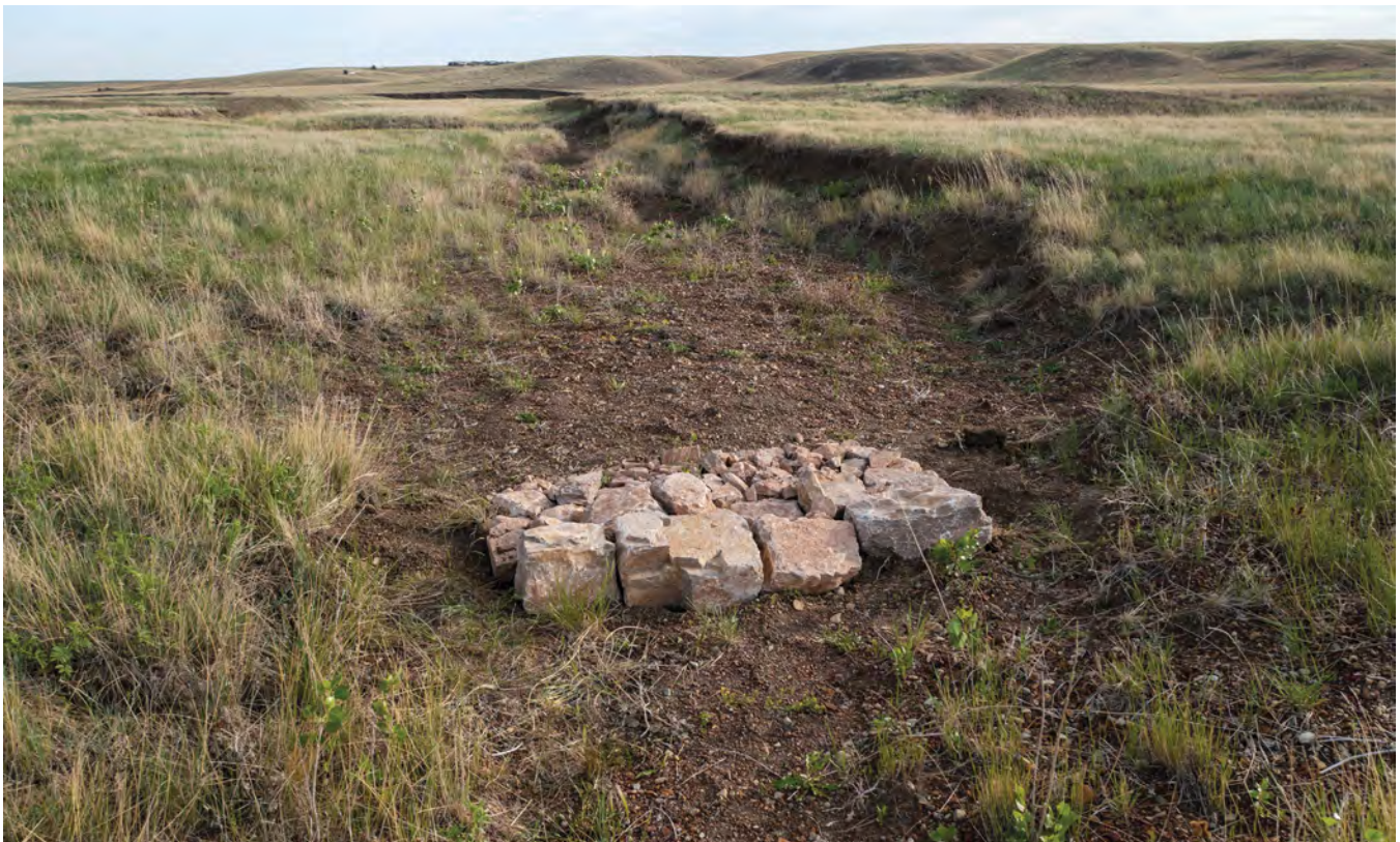
Figure 4. An example of a rock structure installation in one of the dry stream channels on Boylan's ranch. These structures will act like speed bumps for flowing water, slowing it down to reduce erosive energy and helping to trap sediment. Photo © Joe Dickie, Generation Photography, Inc.
