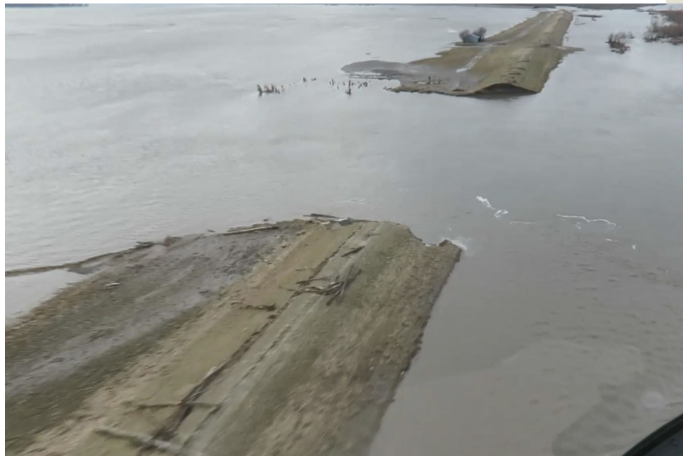
One of the five L-536 breaches in Atchison County, MO, in 2019.
